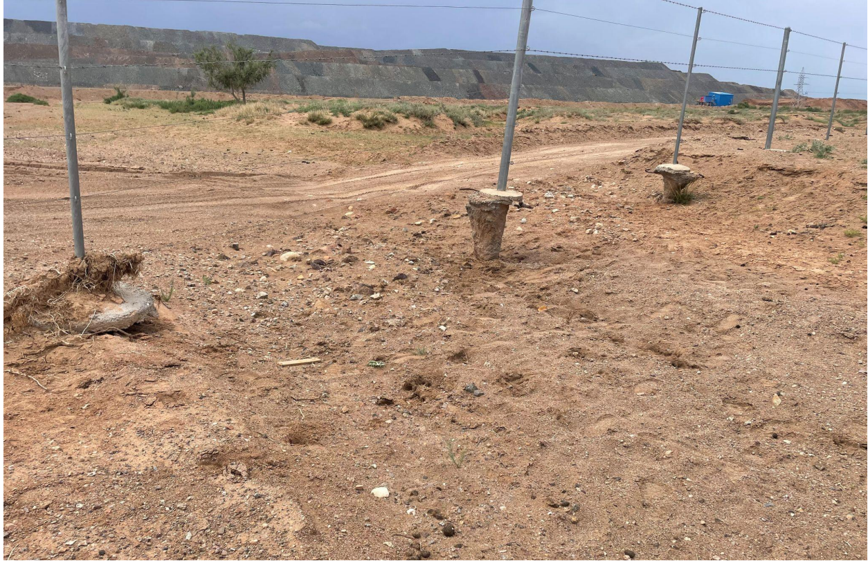
Photo taken by AC on 22 July 2023 showing the current state of erosion along the drainage channel.
