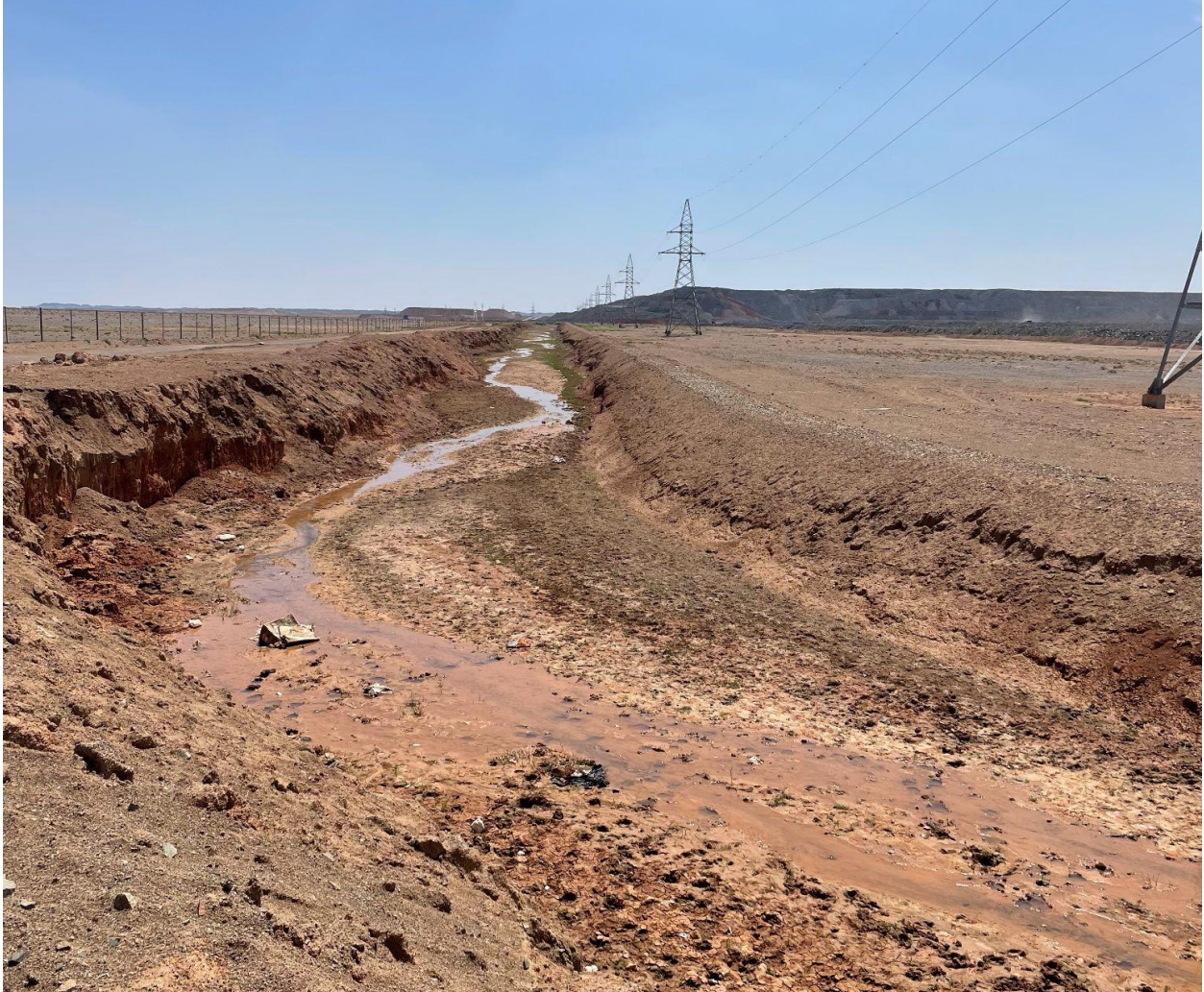
Photo taken by AC on 22 July 2023 showing the current state of erosion along the drainage channel.
